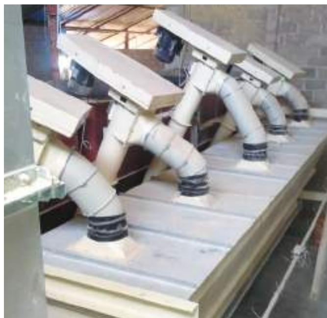
Weighing with automatic feed supply from raw material bins in Nasarawa State, Nigeria. (Image: Alvan Blanch)
